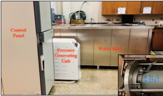
Figure 5: Hydrostatic Pressure Testing Equipment
